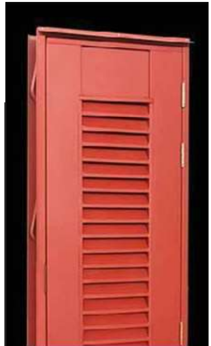
Transformer Room Doors
